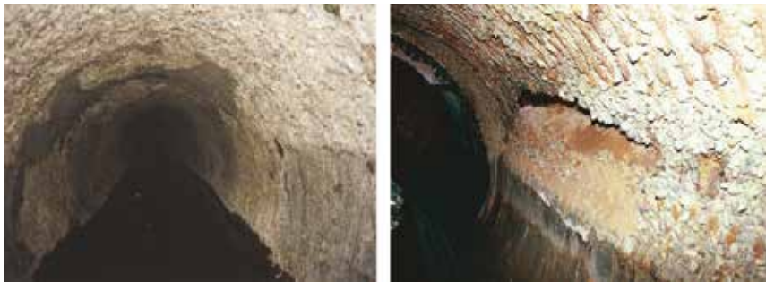
Figure 3.1. The condition of Industrialnyi area sewer tunnel in Kharkiv
