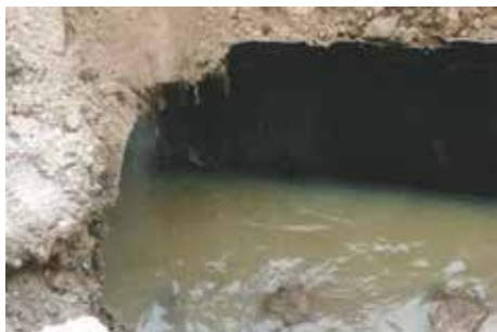
Figure 3.3. A 1,500 mm diameter sewer deteriorated due to corrosion on Pivdenna street in Kharkiv
