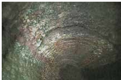
Figure 3.2. Corrosion of the walls of the 2,000 mm diameter sewer tunnel on Matrosova street in Kharkiv
