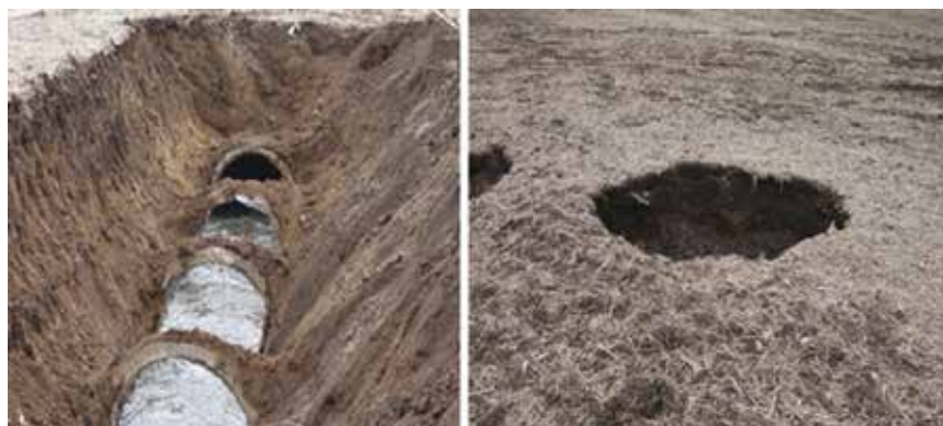
Figure 3.4. A collapsed sewer at Bezlyudivski treatment facilities
