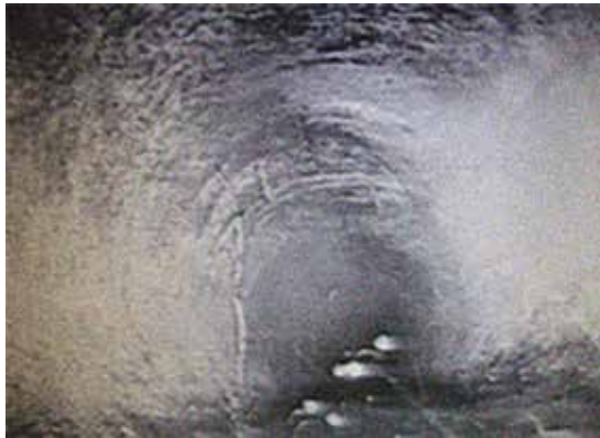
Figure 6.3. Teleinspection of the sewer on Frunze Prospekt after cleaning using the method proposed by the author (RF1, Kharkiv, Ukraine, 2017)
