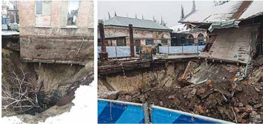
Figure 6.8. Soil failure due to the accident in the reinforced concrete tunnel; and disruption of the bearing capacity of the adjacent house due to local damage to the vault of the tunnel
